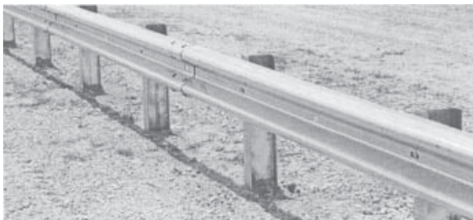
Fig. 1. Guardrail placed along roads
